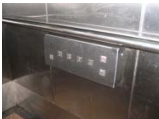
Photo 2-5-3 KL Sentral Station elevator (1)
